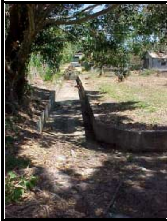
Figure 4. The northern edge of the drain in the middle of the partially formed lane, looking south with the proposed Parks Street precinct on the right of the drain and photo
